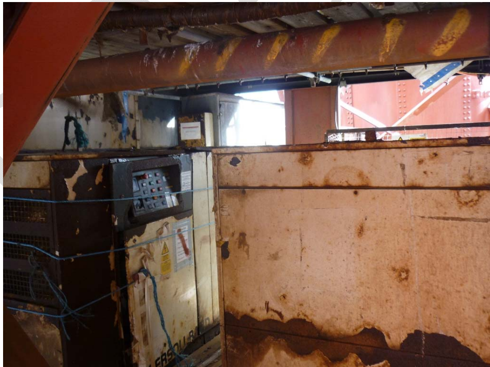
Compressor and interior of housing
